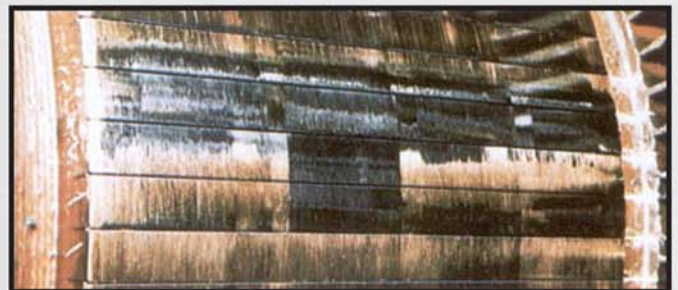
Figure 7 Pitch Bar Burning – Commutator bar burning is a regular pattern caused by a cyclical mechanical or electrical disturbance.
